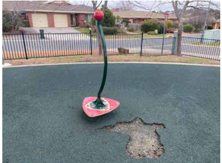
Request > Repair hole in soft rubber flooring
